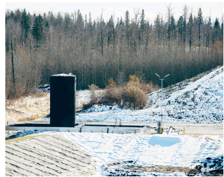
Leachate collection tank at SECURE's Pembina Landfill
